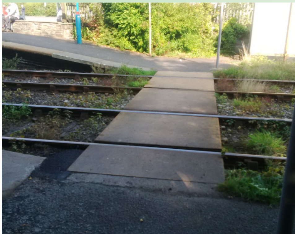
Figure 18: Llanwrtyd – pedestrian foot crossing providing step-free access between platforms – but without warning lights or barriers
