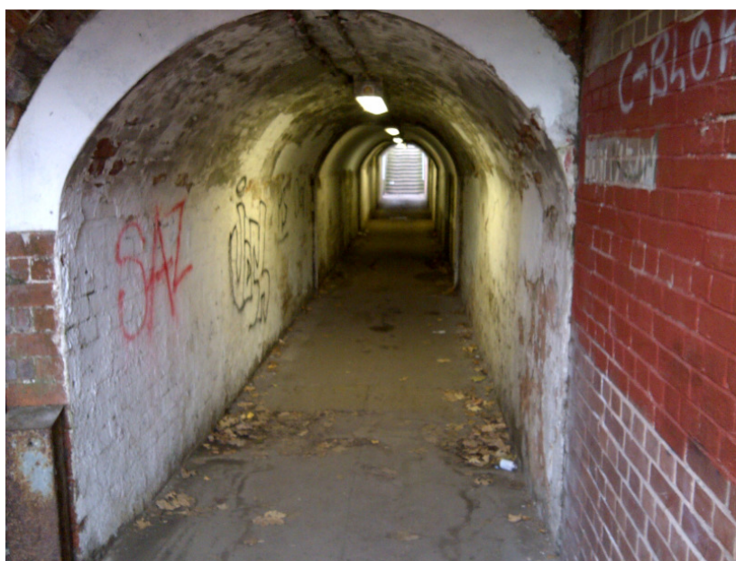
Figure 31: Access subway to Retford station – an environment likely to make many people feel unsafe
